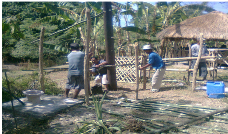
Figure 2: Photo of the purok members renovating their dap-ayan and building other facilities around the dap-ayan . (January 2011)
